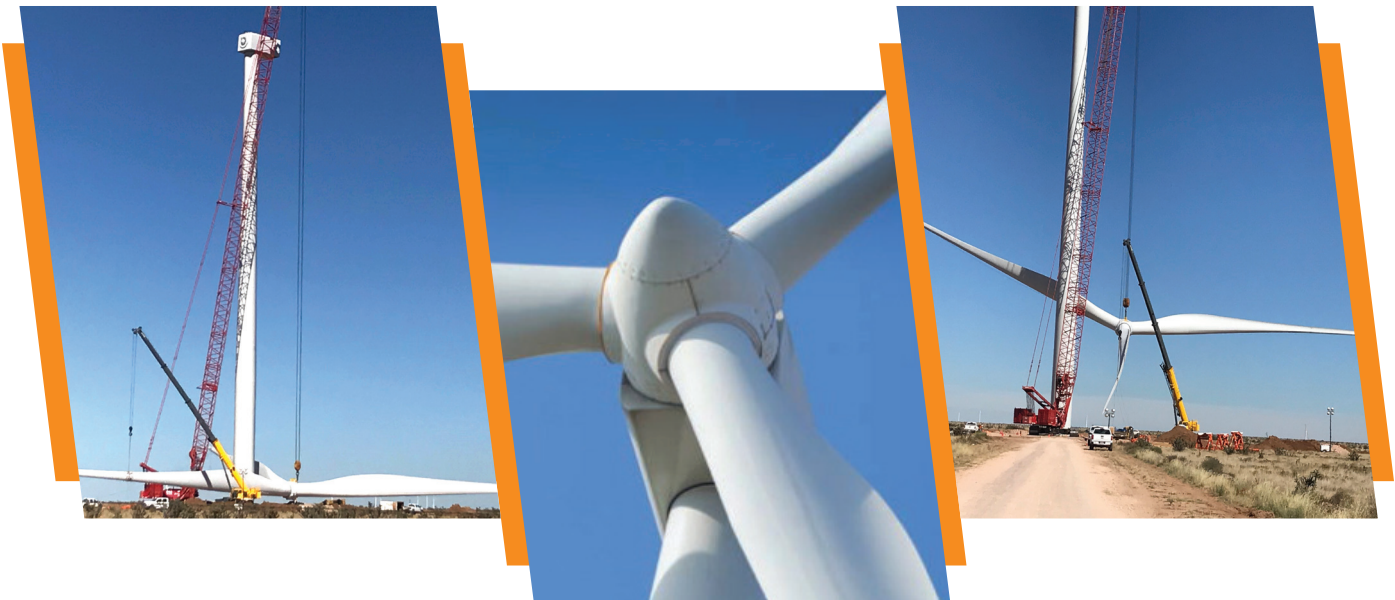
Crews install a wind turbine at the NextEra Energy Resources wind facility near Santa Rosa.
