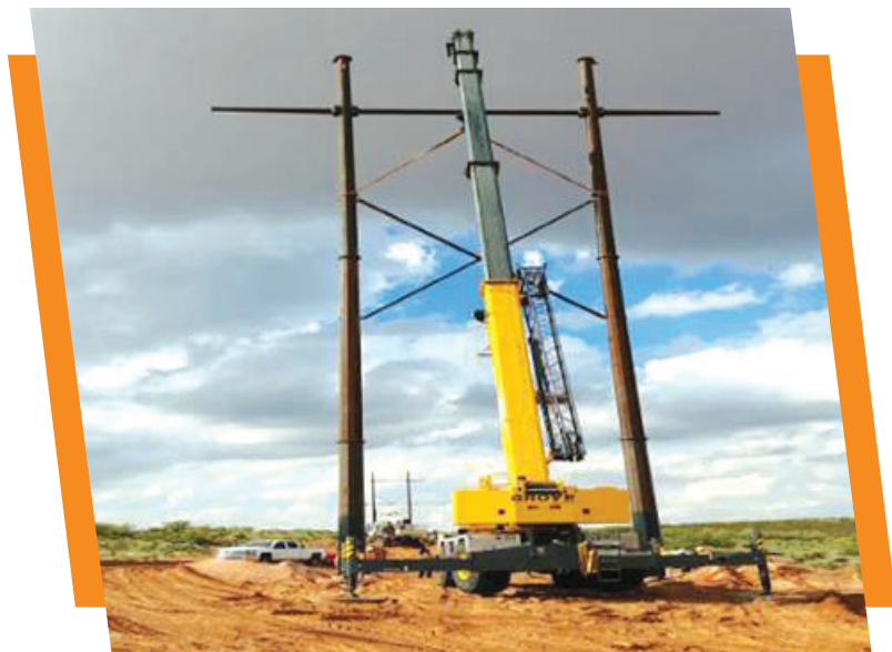
Construction begins on SPS's $400 million transmission project. The 86-mile, 345-kV transmission line between Hobbs and the China Draw Substation, southeast of Carlsbad, will provide the power necessary to sustain industrial growth and job creation in southeastern New Mexico.
